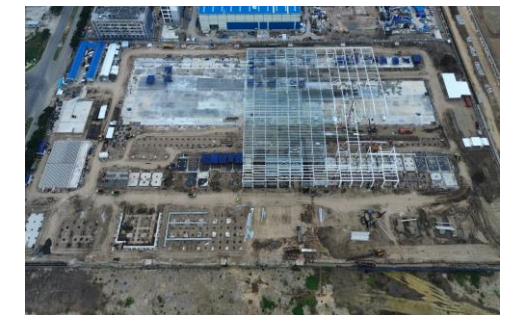
Solar PV Manufacture (Kendal)
