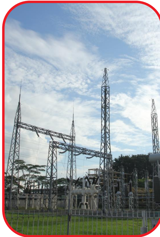
Power and Steam Generation
