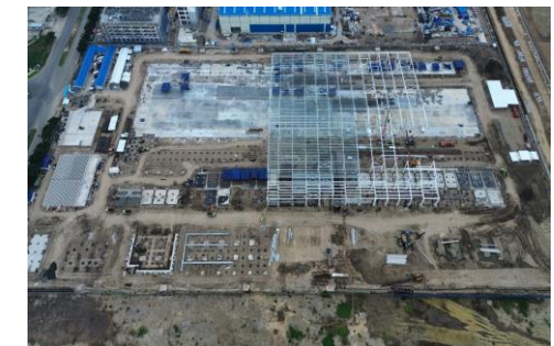
Solar PV Manufacture (Kendal)
